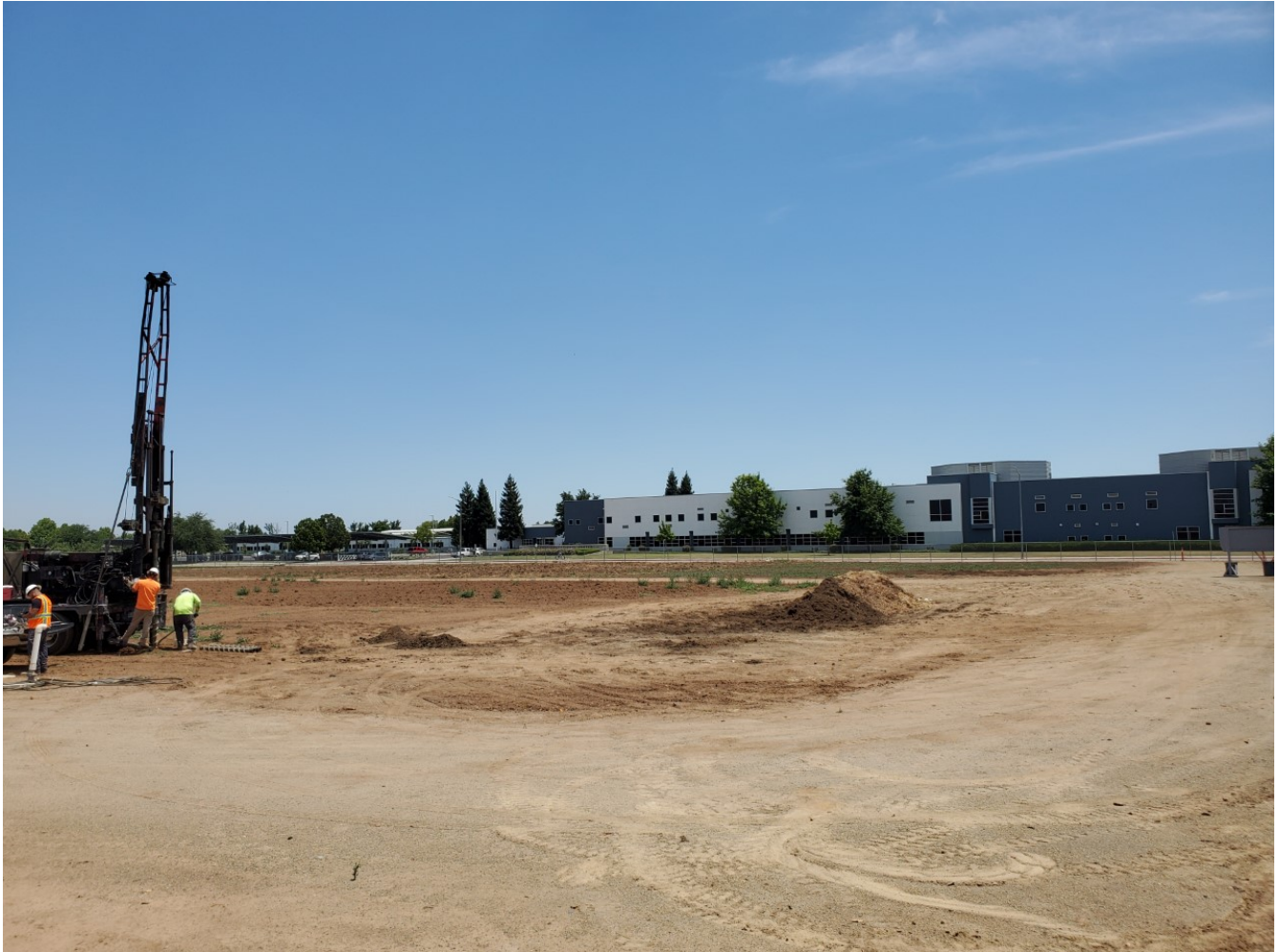
Photo of the area where the new CTE building will be constructed. Photo taken on June 11, 2020.
