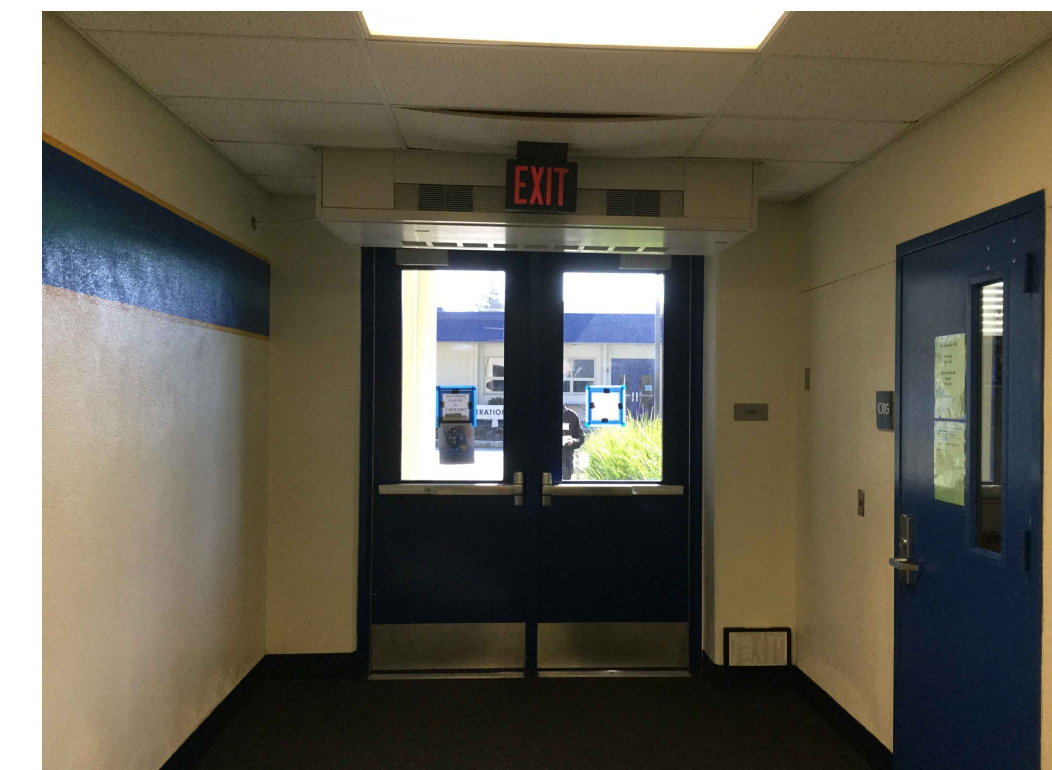
INTERIOR DOOR # C1, C2, C3, C4, C5
